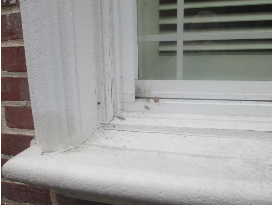
Original wood contains lead based paint
