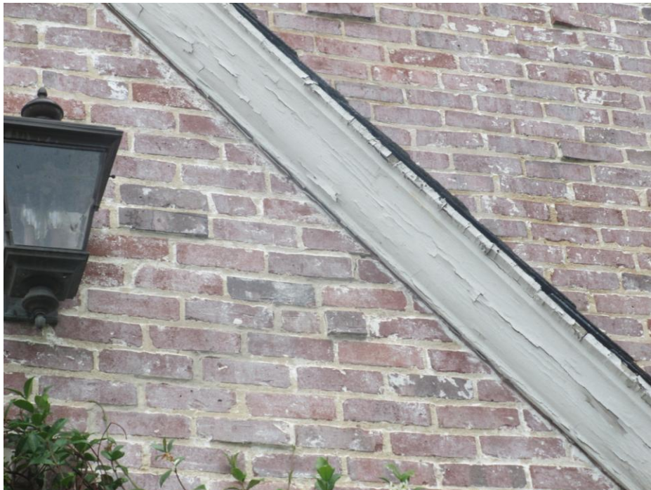
Fascia contains deteriorated lead based paint and is a hazard.
